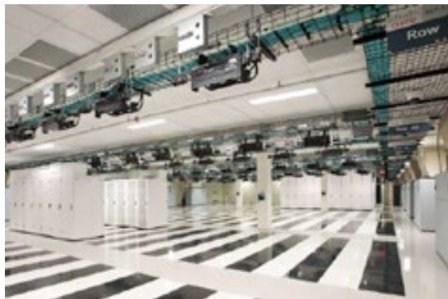
Cisco data center, Research Triangle Park, North Carolina
